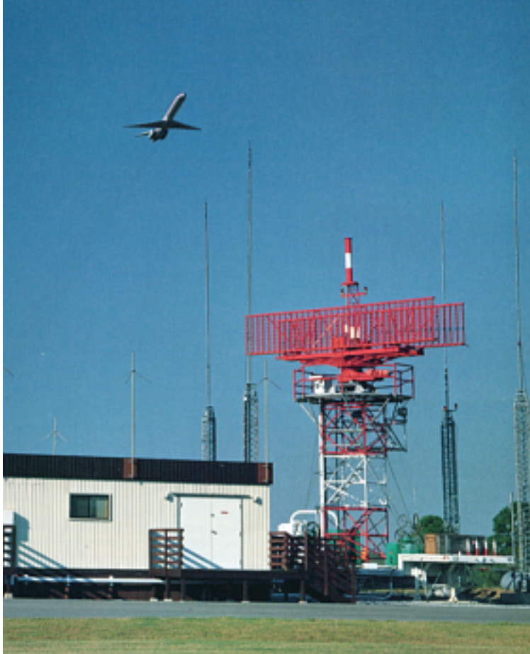
Figure 6.2: Mode S Ground Station and Antenna
